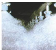
Desulfurization Tower Spraying Of Power Plant
